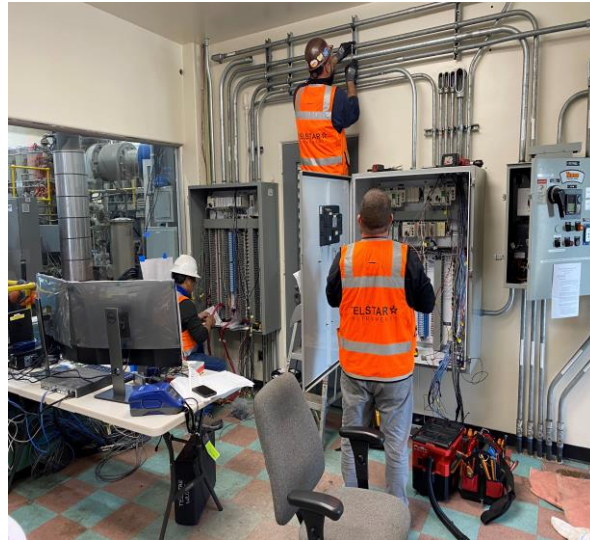
Supervisory Control and Data Acquisition System (SCADA) Installation at Ettie Street Pump Station
